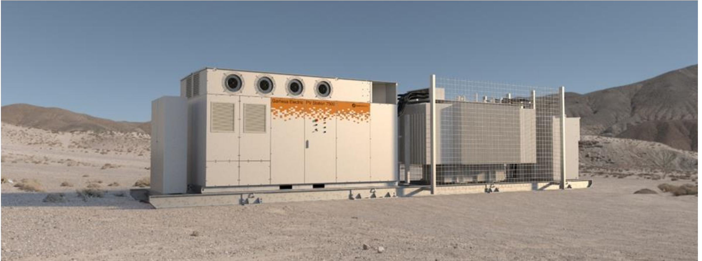
Gamesa's new PV Station (up to 7.5MW) including MV transformer and switchgear.
