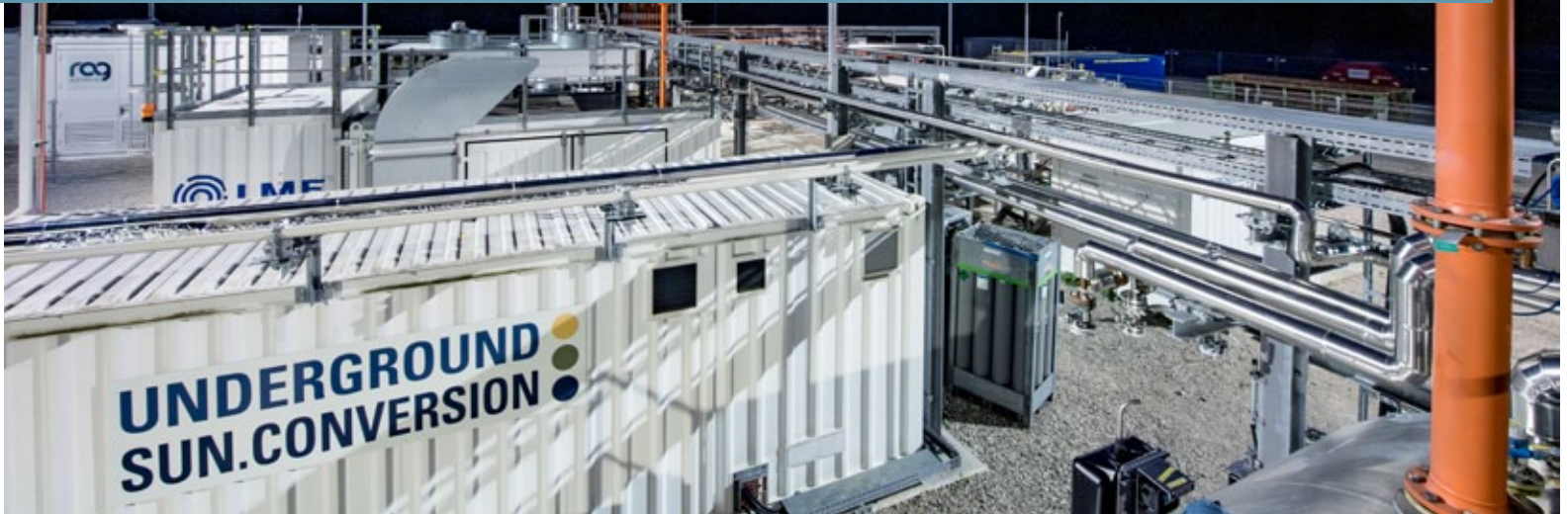
RAG-Anlage in Pilsbach/Oberösterreich Foto: RAG Austria AG/Karin Lohberger Photography
